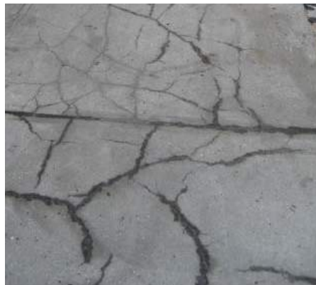
Broken and unmaintained sidewalk paving is arguably inaccessible, an eyesore and creates a perception of an "unkept & uncared for" area.
